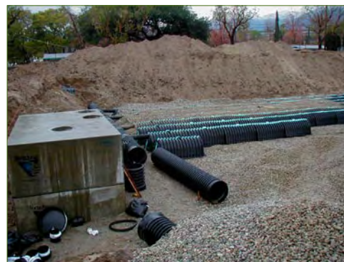
Two hundred and twenty infiltrator units below the ball field hold up to 95,200 gallons of water.
